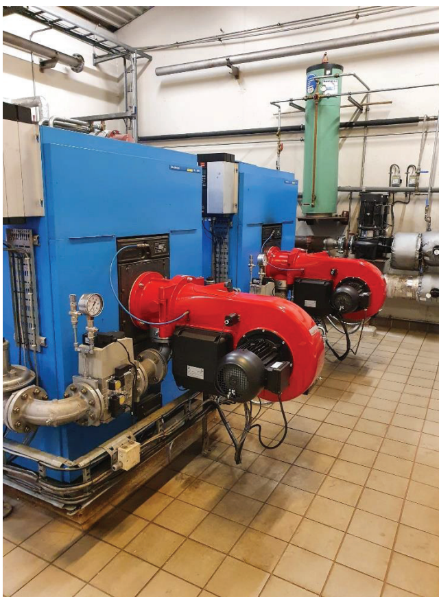
Oppgradering biogass anlegg
