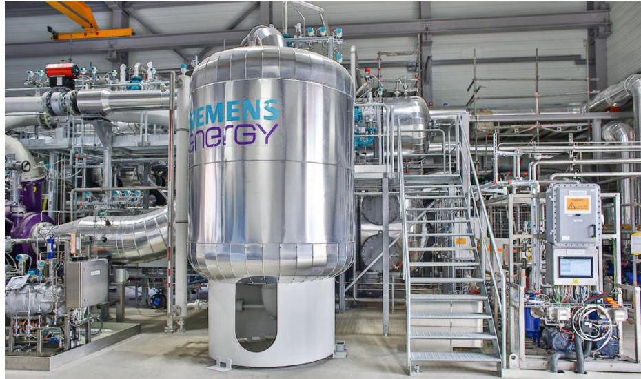
District heating system, MVV / GKM Mannheim, Germany
